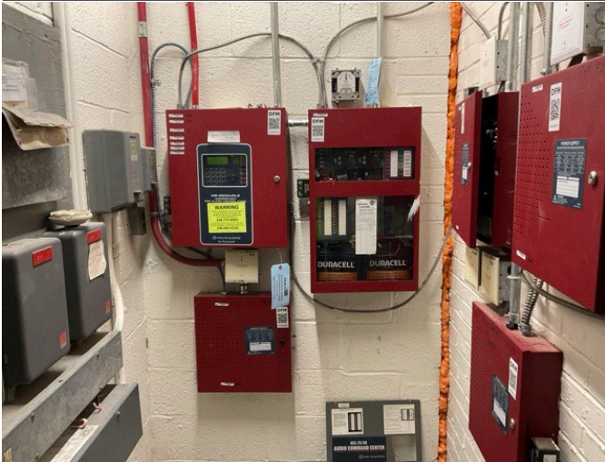
19 - FIRE ALARM PANEL
