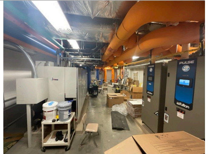
8 - NEW BOILER ROOM
